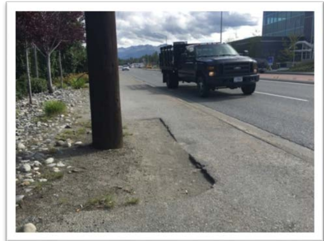
FIGURE 10. OBSTRUCTION IN SIDEWALK ON 36 TH AVENUE
