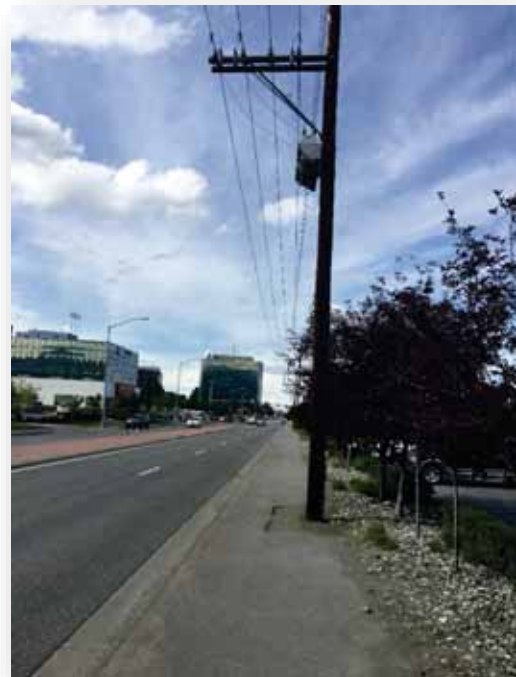
Figure 13: ML&P overhead utility
